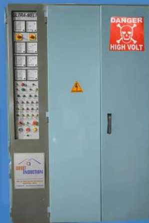
Induction Furnace Power Supply
